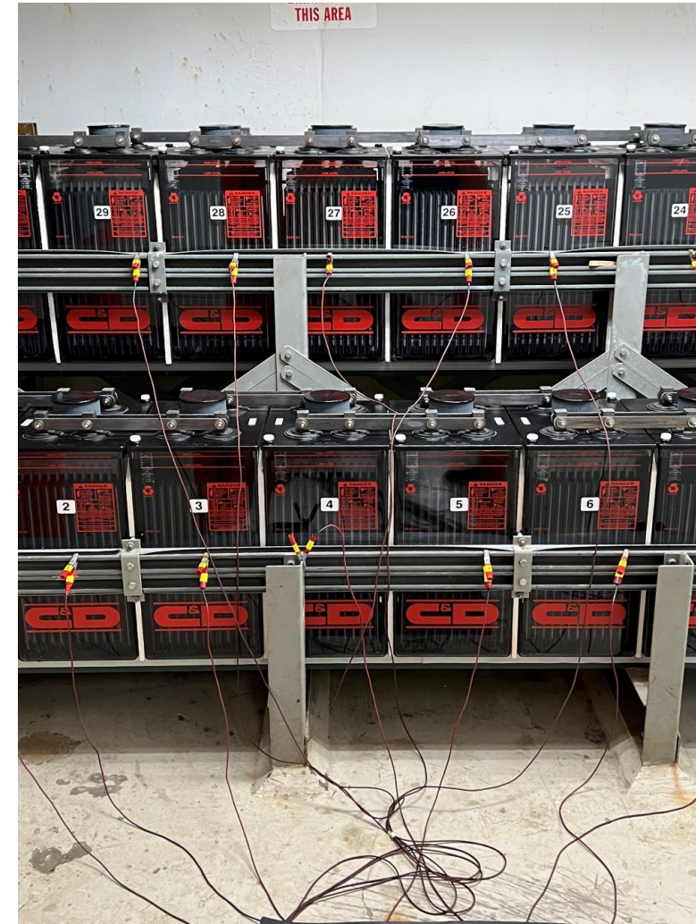
Non-Vital Battery 1-6 with Test Leads Installed
