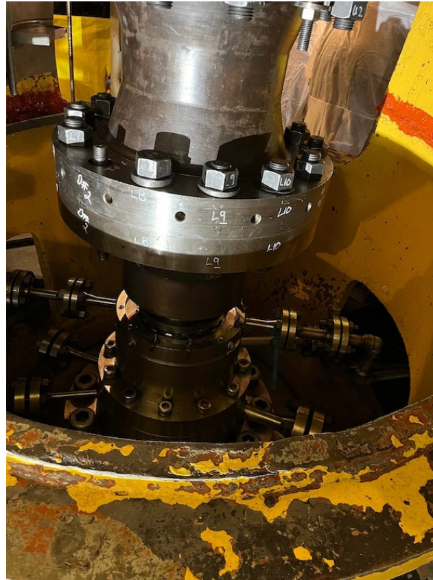
Reactor Coolant Pump Seal
