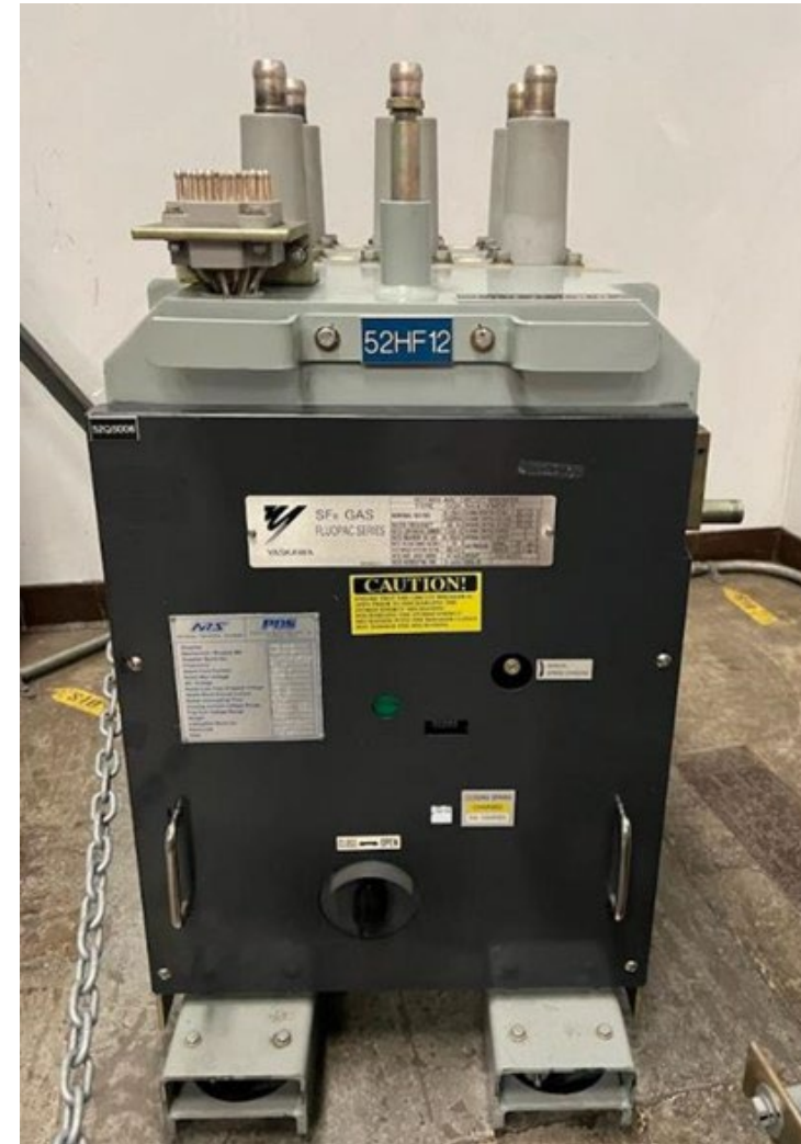
Spare 4kV Breaker
