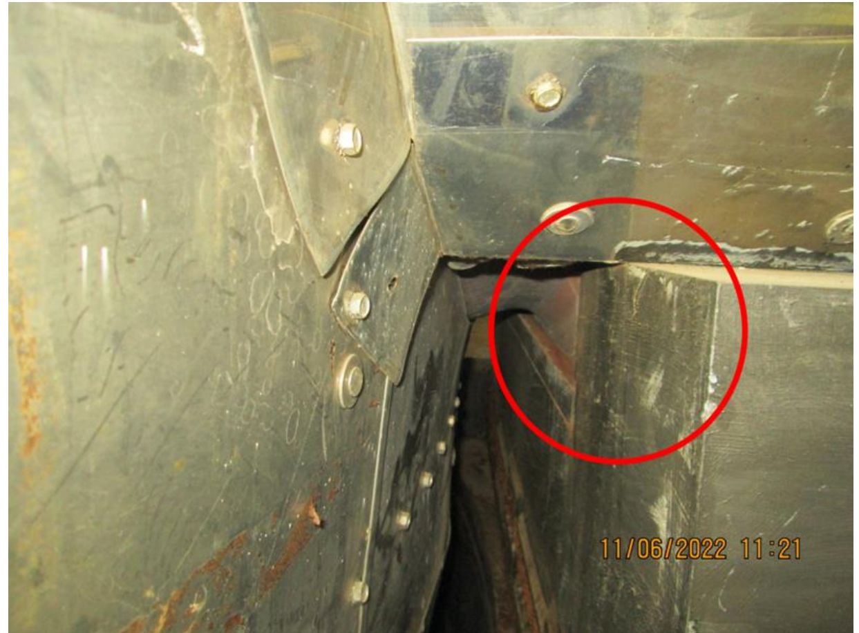
Steam Generator and Reactor Vessel Supports
