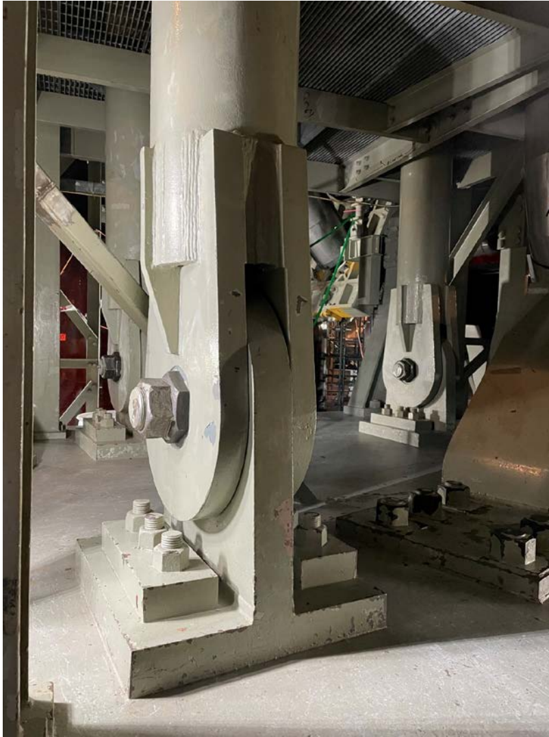
Picture 3.10-4, Steam Generator Support Legs
