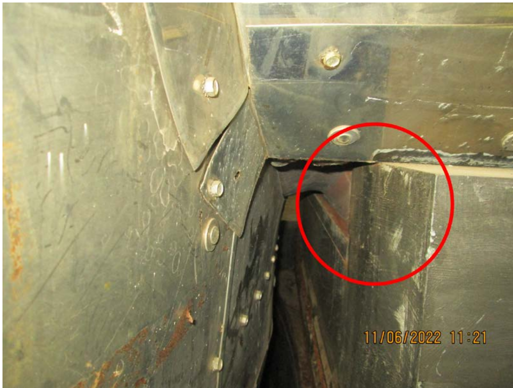
Picture 3.9-1, Reactor Vessel Support Under Loop 3 Cold Leg. Note the horizontal restraint to motion during earthquakes (circled).
