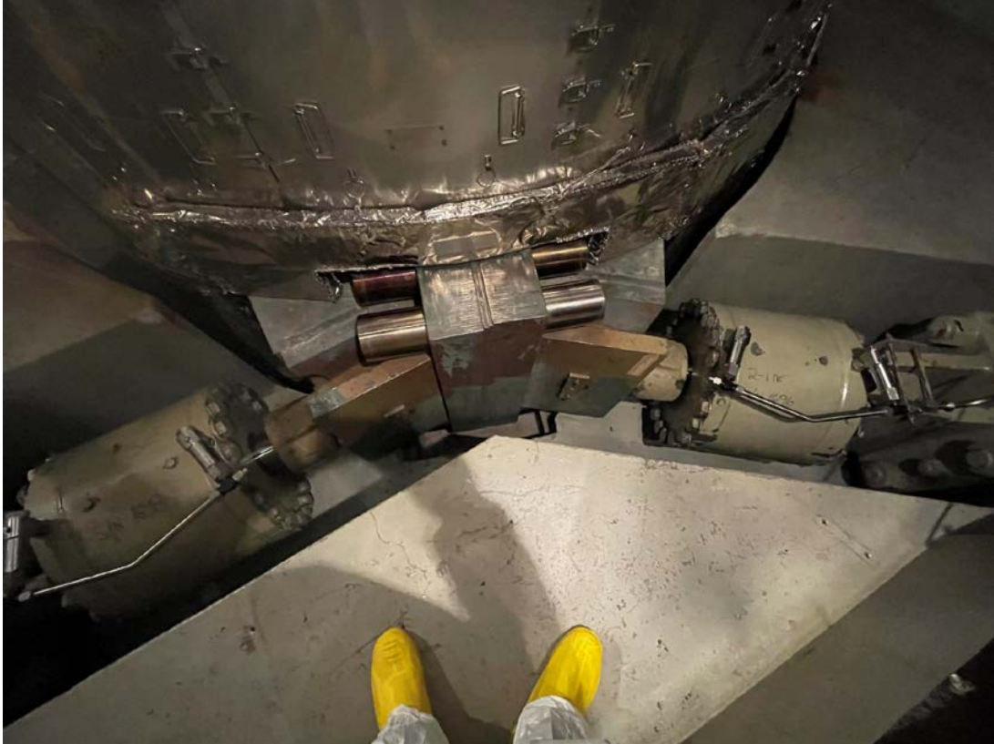
Picture 3.10-2, Large Bore Hydraulic Snubbers (Steam Generator Lateral Supports)
