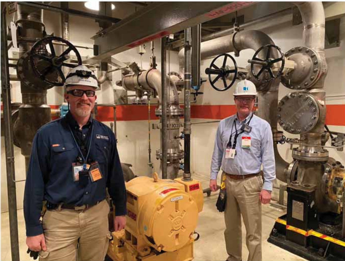
System Engineer and Dr. Peterson at SFP Cooling Pumps
