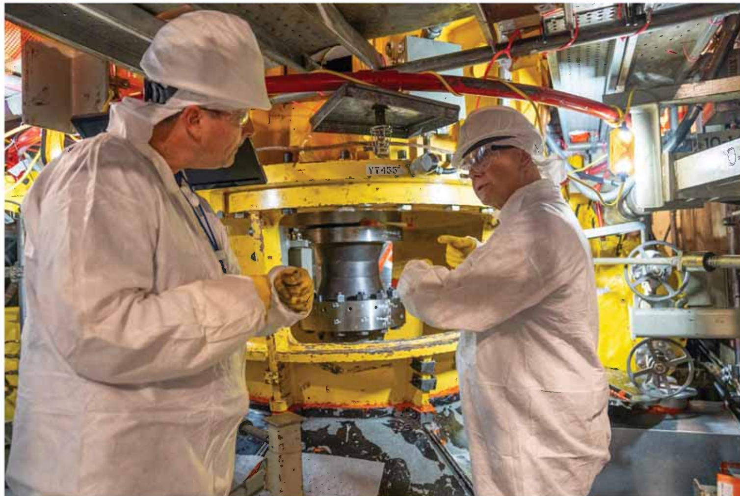
Mr. Soenen and Dr. Meshkati at Reactor Coolant Pump 1-3 Motor/Pump Coupling
