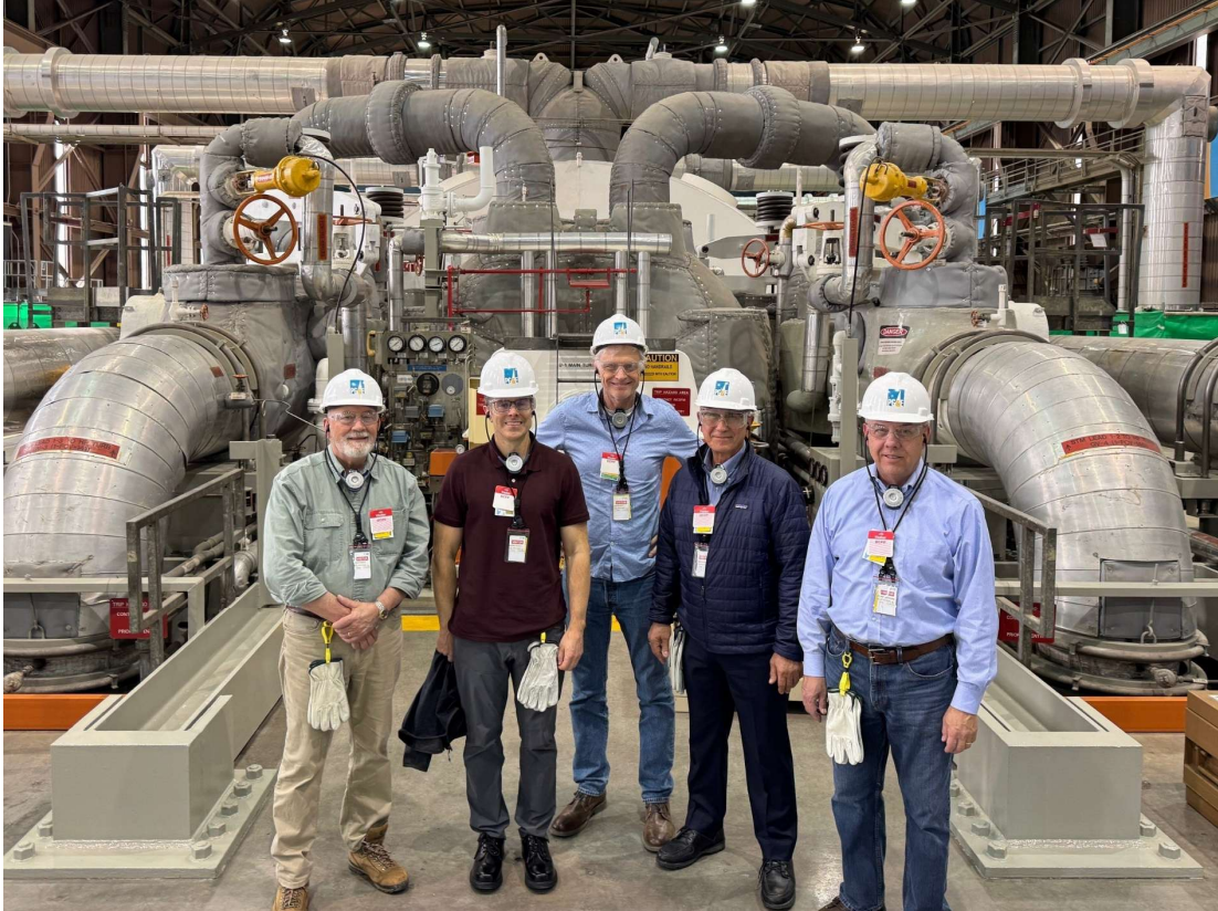
SRT and FFT at Unit 1 High-Pressure Turbine
