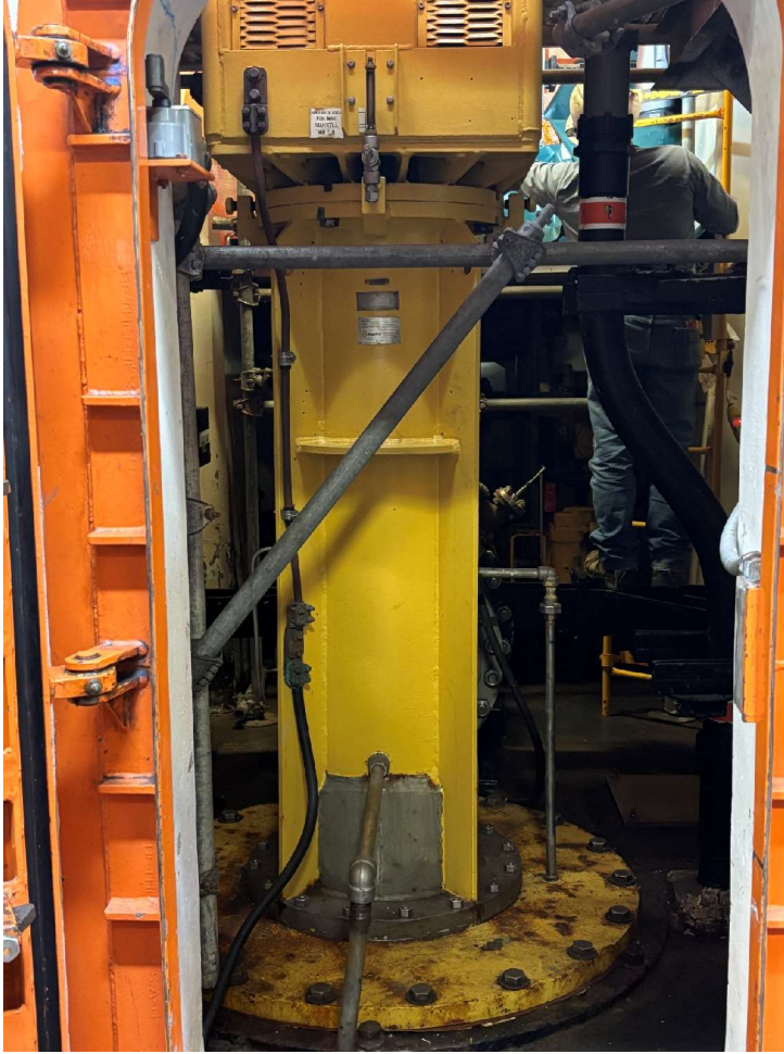
Auxiliary Saltwater Pump 1-1
