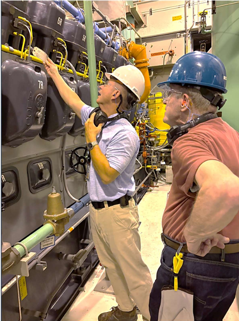
Mr. LaChance and Dr. Budnitz at the 2-2 Emergency Diesel Generator
