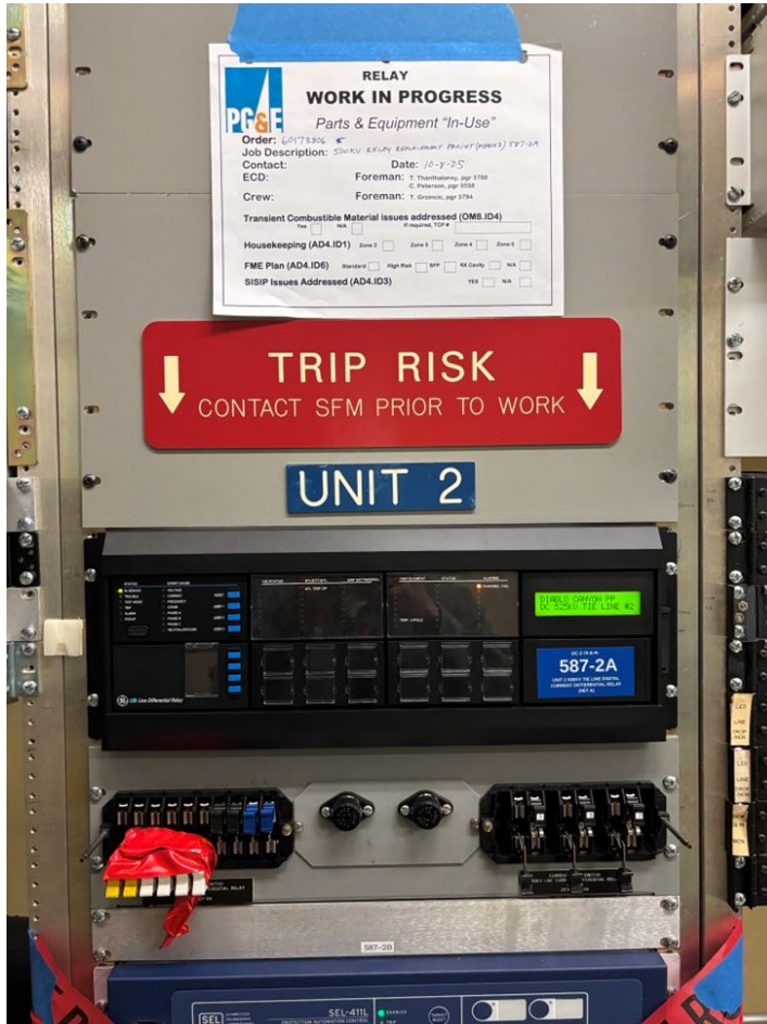
500kV Tie-Line Relay Upgrade
