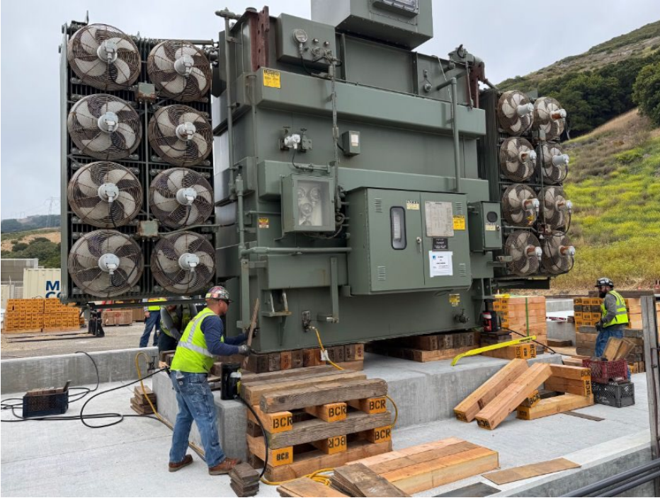
Transformer Radiators (behind fans)
