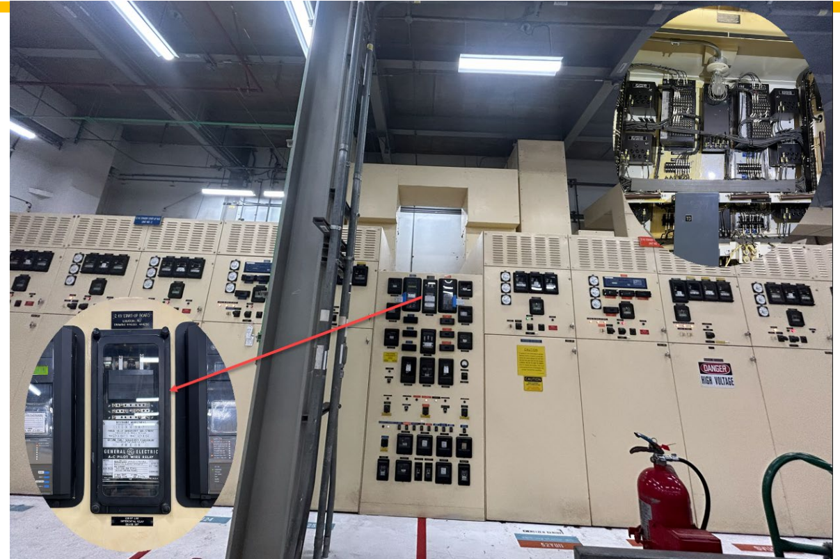
230kV Relay Replacement (with digital Switcher )
