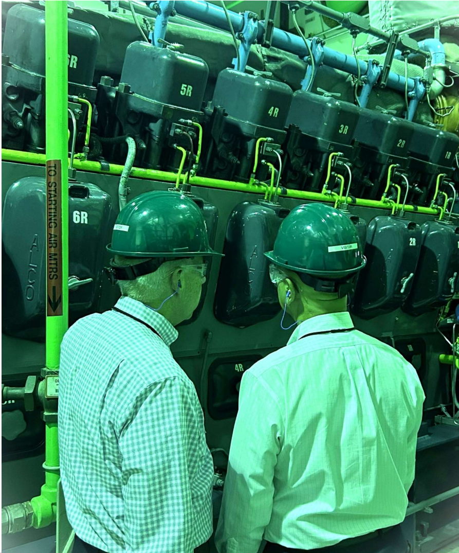
Mr. McWhorter and Dr. Meshkati at Emergency Diesel Generator 1-3
