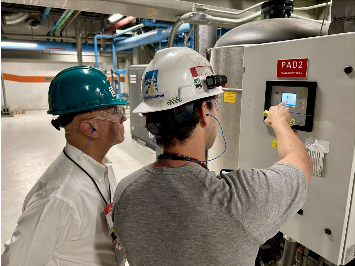
Dr. Meshkati and Mr. Mahoney Observing Operating Indications on a Plant Air Dryer
